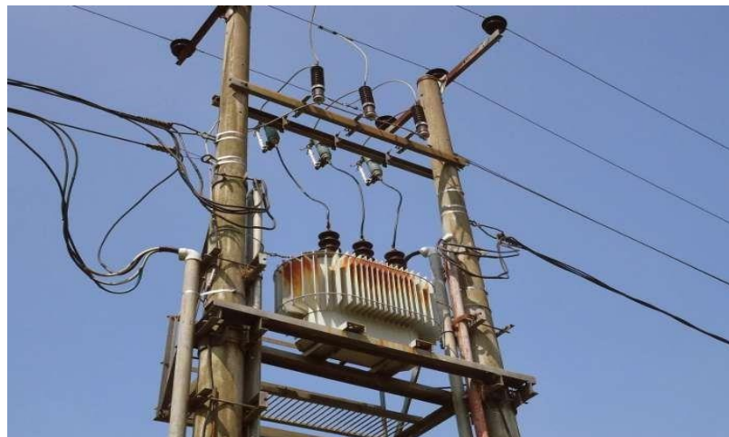
Gambar 2. 3 Transformator Distribusi Sumber : ( https://rakhman.net/electrical-id )
