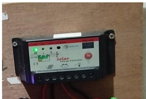
Gambar 2.1.2 Solar Charge Controller tipe PWM.
