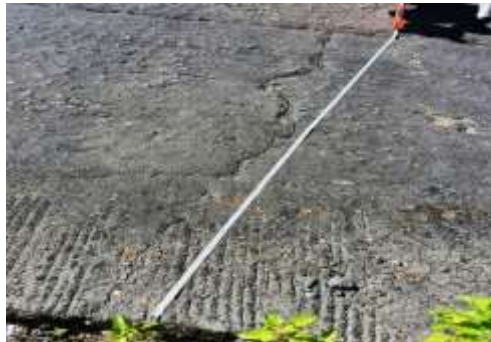
Linear Cracking (m)
