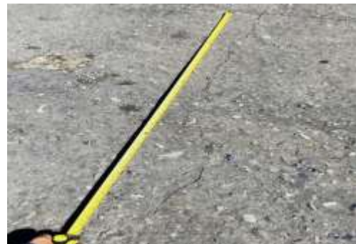
Shrinkage Crack (m)
