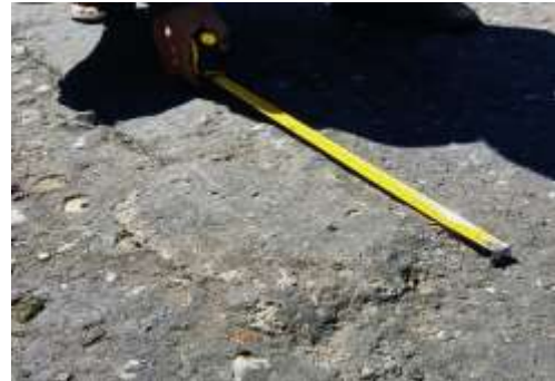
Patching Small (m 2 )
