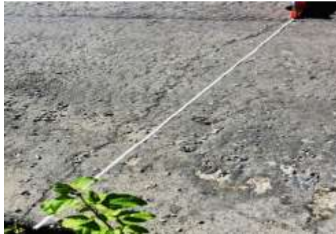
Linear Cracking (m)
