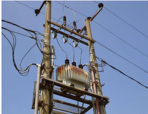
Gambar 2. 7 Transformator Distribusi Sumber : ( https://rakhman.net/electrical-id )
